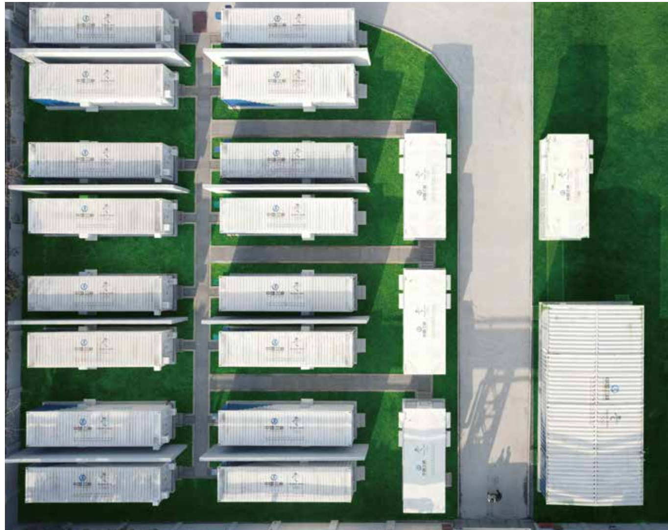
10MW/39MWh Energy Storage Station
