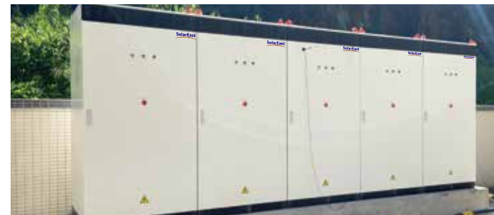
Industrial & Commercial Energy Storage Project, Guangdong
