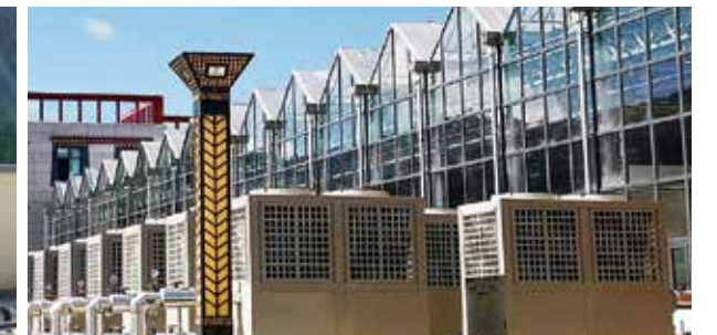
Heat Pump Project, Jingtu Industrial Park in Caina Town, Tibet
